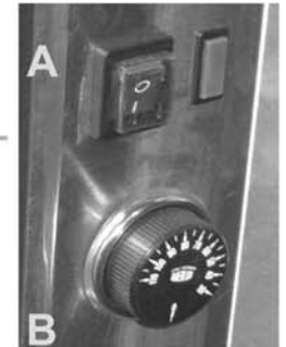
Hot Cupboard Controls
